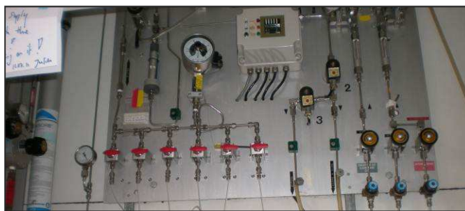
Photo 2: Station de gaz
