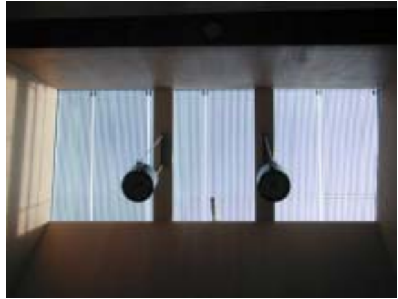
Figure 23: PV shading installation Würth, view of the inside, Chur (Photo: NET)
