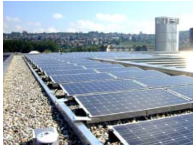
Figure 29: 47 kWp IBM flat roof installation, Zurich (Photo: NET)
