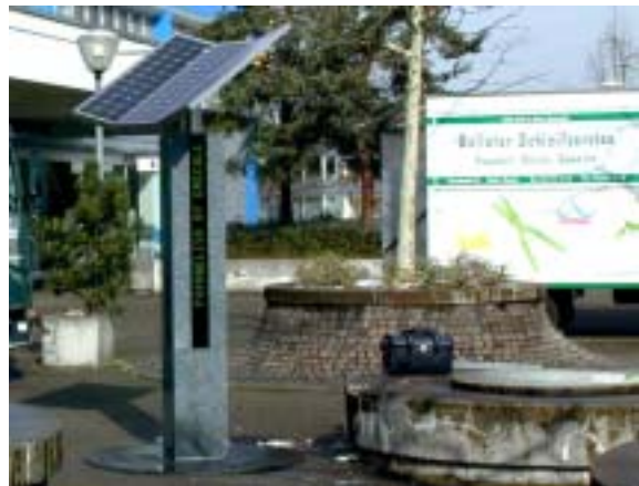
Figure 27: Stand-alone photovoltaic Obelisk, Zurich (Photo: Enecolo)
