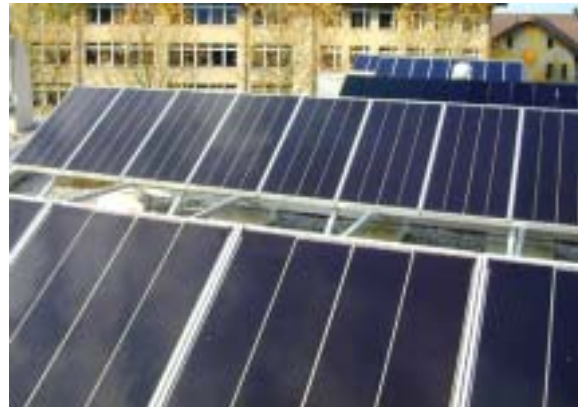
Figure 37: 3x1 kWp Newtech test installations in Burgdorf (Photo: NET)
