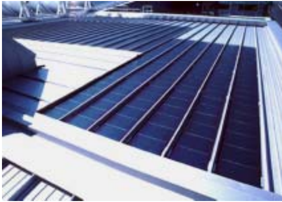
Figure 32: 3 kWp PV Eurodach with amorphous cells (Photo: NET)
