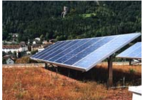
Figure 33: 10 kWp Solgreen green roof installation in Chur (Photo: NET)
