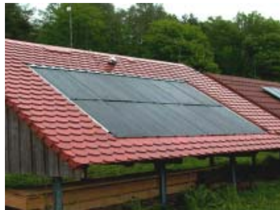
Figure 5: Outdoor demonstration facility for testing CIS elements in the HIPERB project (photo: 3S)
