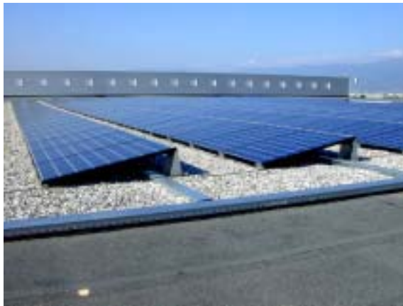
Figure 24: 70 kWp Palexpo flat roof installation in Geneva (Photo: NET)
