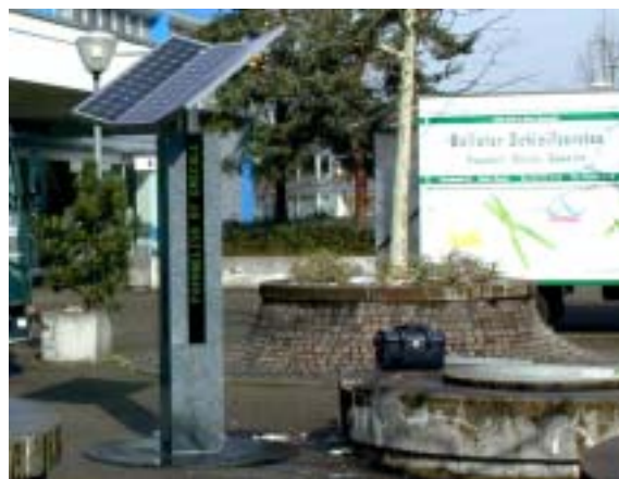
Figure 27: Installation photovoltaïque autonome Obelisk, à Zurich (Photo: Enecolo)
