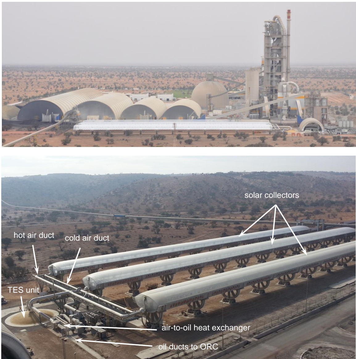
Figure 1: Aerial views of the CSP pilot plant construction site (Courtesy of Italcementi group).
